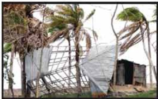
The wind is blowing the roof away.
